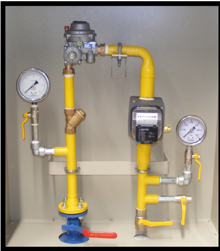
Metering skid with RPD Flow Meter
