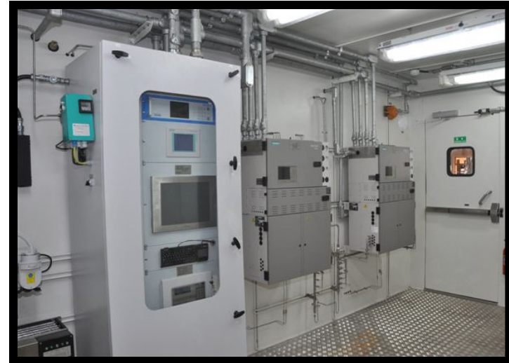
Analyzers inside Analyzer House
